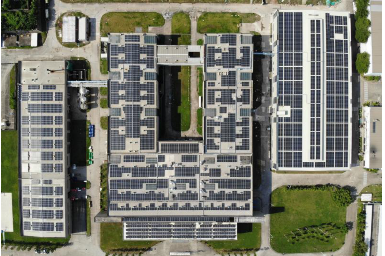
Solar panels have been installed on all roofs of ECCO Tannery Xiamen since 2019
