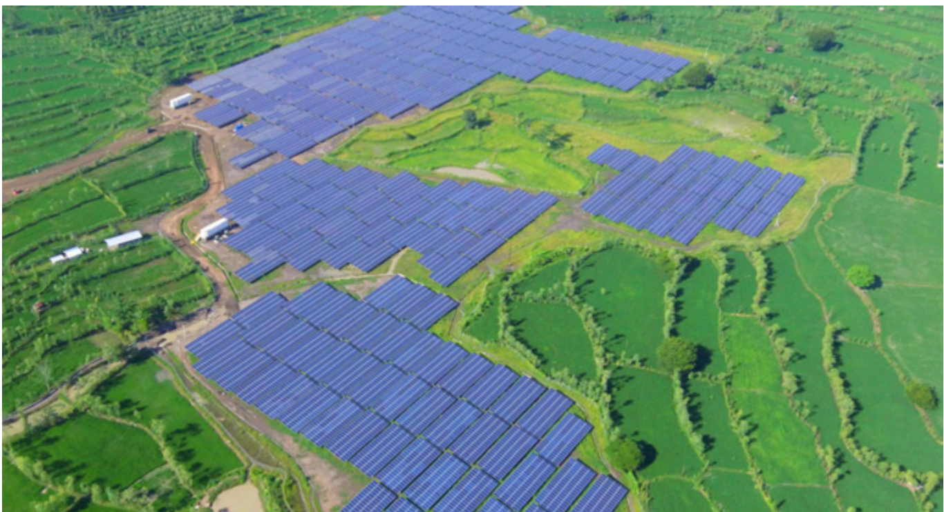
Solar panels in Sulawesi, Indonesia. (Photo: Rumagja Bangun Setiawan)
