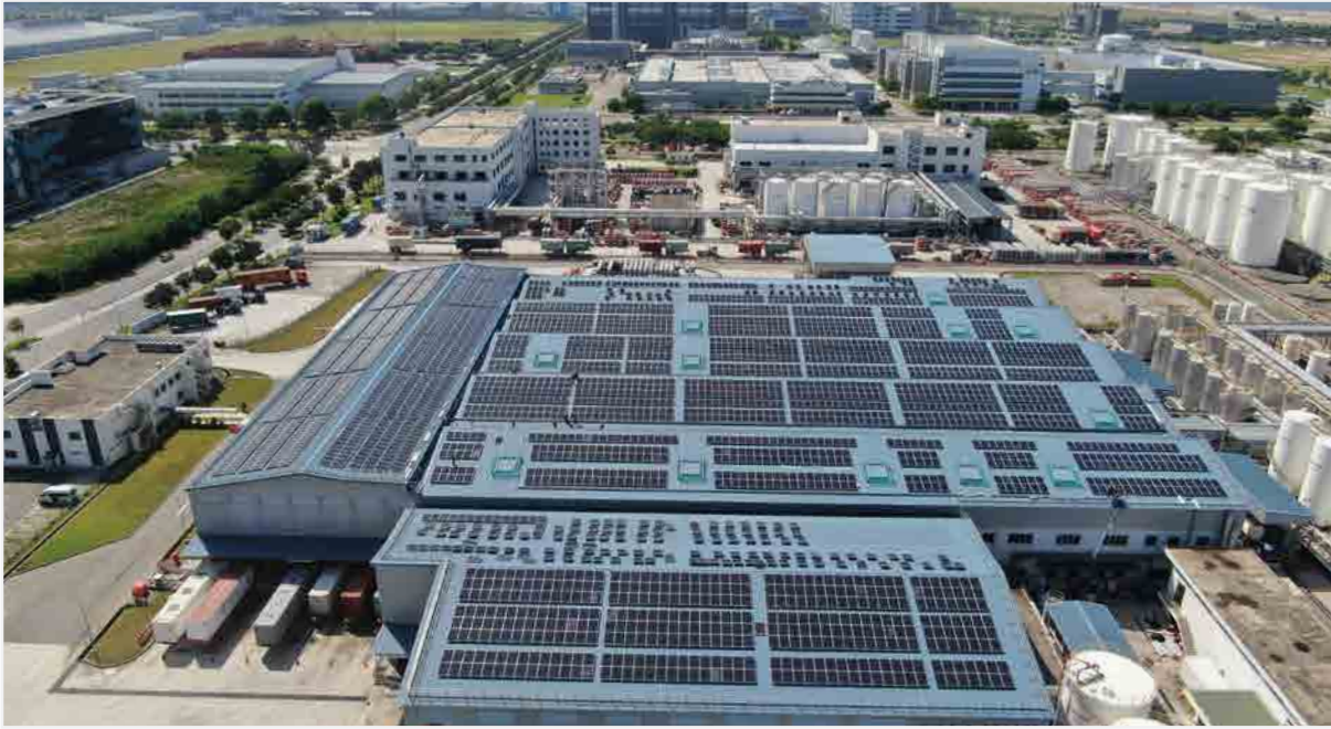
Total lubricants plant in Singapore solarised by Total Solar DG Southeast Asia
